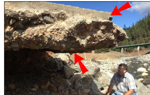
flood water undercut launching ramp
