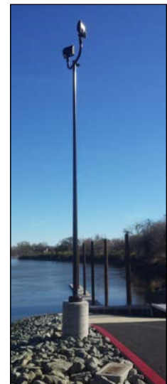
launch ramp lighting
