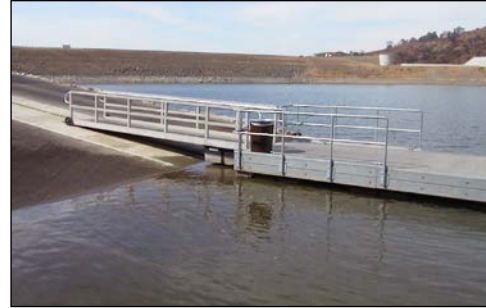
gangplank access to boarding floats
