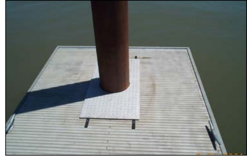
sliding pile yoke cover on round pile
