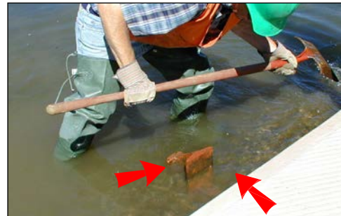
precast panel is nearing catch cleat as worker clears away plowed gravel
